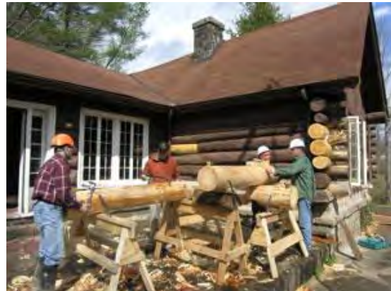
Rehabilitation work at the Putney Ranger Station, originally constructed in the 1930s by the Civilian Conservation Corps, Harlan County
