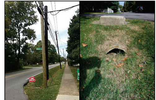
Figure 8: Utility Poles in Ditches (left) and Silted Pipe (right)
