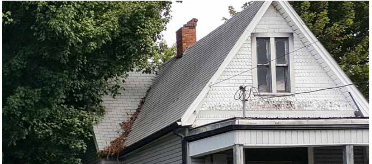
Note leaves in valley, missing bricks at chimney and overhanging limbs
