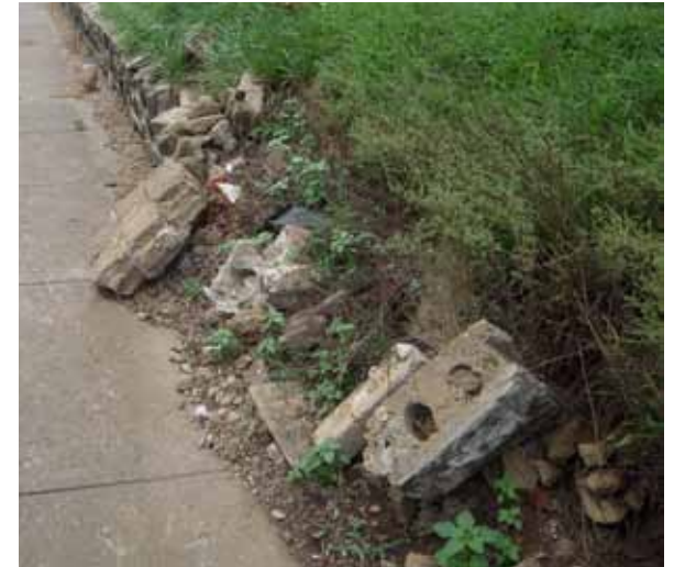
Failing retaining wall along SR 64
