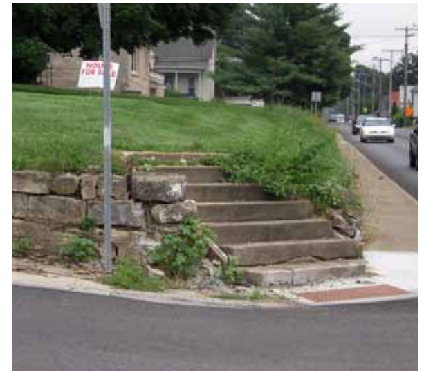
Failing retaining wall and steps along SR 64
