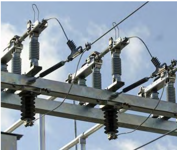
Power Conversion Utility Example
