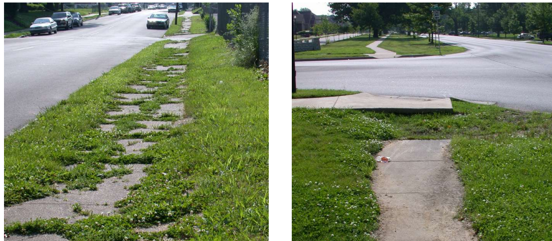
Figure 9: Sidewalks may become hazardous or inaccessible if not properly constructed and maintained. The sidewalk on Muhammad Ali Blvd at Southwestern Pkwy is cracked and becoming overgrown (right). New and old sections of sidewalk along Algonquin Pkwy do not line up (far right).
