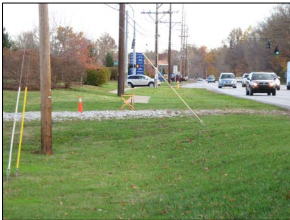
Looking eastbound on US 42 at the proposed tie in at the existing sidewalk stub just west of the Timber Ridge Drive intersection.
