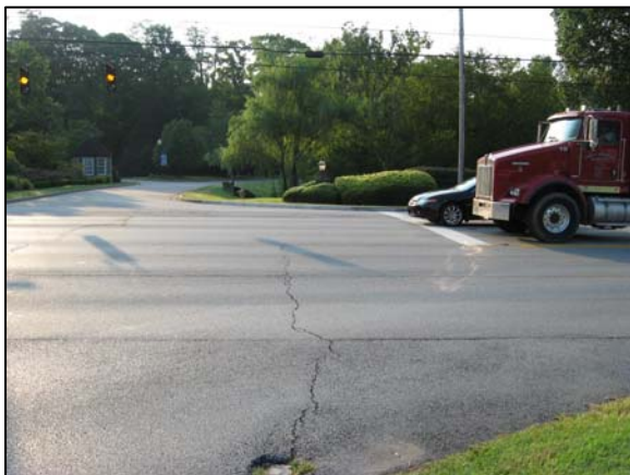
Looking south at the Fox Harbor Road and US 42 intersection from Prospect Point.
