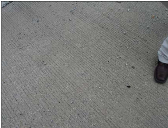
Debris on Shoulder of KY 1526
