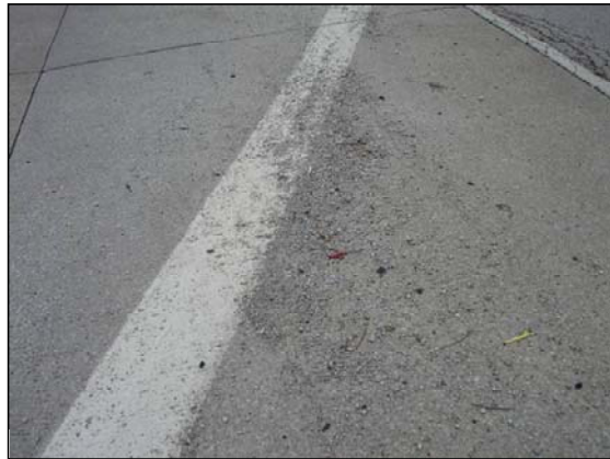
Debris in Island Next to Ramp
