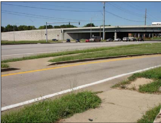
Southbound Bardstown Road On-Ramp to Westbound Watterson Expressway - Sidewalk
