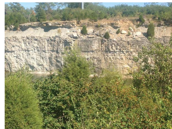
Quarry high wall – flooded pit. Highly erodible and problematic Waldron shale cap.
